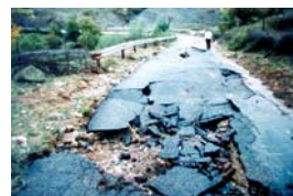
Damages, caused by Varbitsa flooding river
