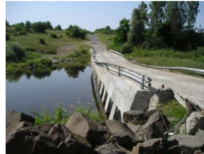
"Flooded" bridge over Plazishte river - the road to village Varhari
